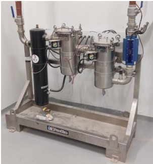
Custom-built fuel polishing systems
